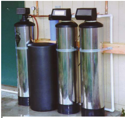
TYPICAL CALCITE NEUTRALIZER (SHOWN ABOVE, STAINLESS STEEL TANK ON THE FAR RIGHT) INSTALLED IN COMBINATION WITH AN IRON FILTER SYSTEM AND WATER SOFTENING SYSTEM
