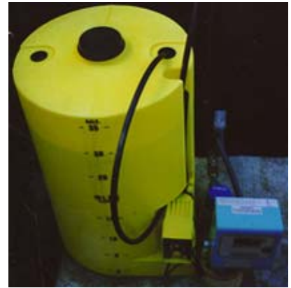
SODA ASH FEEDER - YELLOW SOLUTION TANK (DIMENSIONAL NEUTRALIZER MEDIA FILTER METERING PUMP NEAR WELL HEAD TANK (STORAGE TANK NOT SHOWN))
