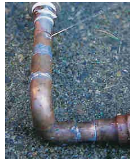
COPPER PIPING CORROSION WITH PIN HOLE LEAKS
