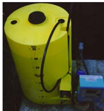
SODA ASH FEEDER. YELLOW SOLUTION TANK (DIMENSIONS: 24" X 36") WITH METERING PUMP, SHOWN INSTALLED NEAR WELL HEAD BEFORE STORAGE TANK (STORAGE TANK NOT SHOWN)
