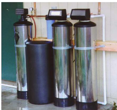
TYPICAL CALCITE NEUTRALIZER (SHOWN ABOVE, STAINLESS STEEL TANK ON THE FAR RIGHT) INSTALLED IN COMBINATION WITH AN IRON FILTER SYSTEM AND WATER SOFTENING SYSTEM
