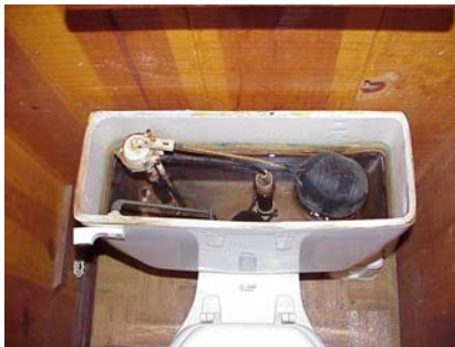
Black or rusty slime, and/or stringy-appearing growths on the sides of toilet flush tanks (above) may indicate the presence of bacterial growth. Water heaters (right) are prime sources of odors when bacteria react with the anode rod inside.
