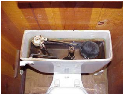
Black or rusty slime in toilet flush tanks (above) indicate the presence of bacterial growth. Water heaters (right) are prime sources of odors when bacteria react with the anode rod inside.
